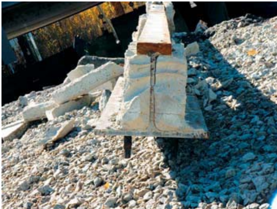
Figure 2: A cross-section of a D-Beam with part of the hollow core planks still attached
